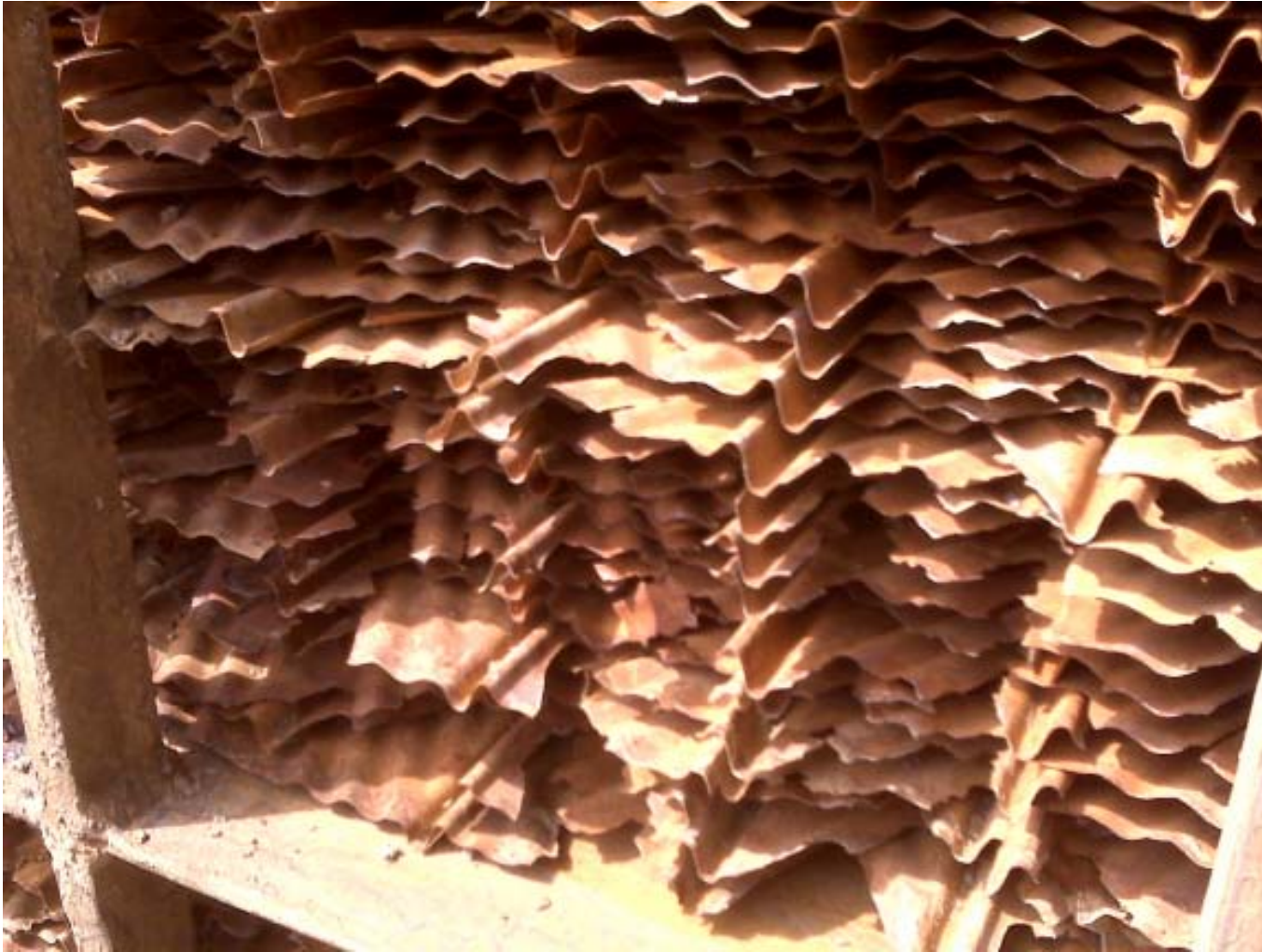
TWO LAYER COLD END DAMAGE
